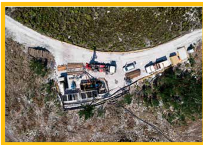
FIGURE 5: Production borehole drilling in progress showing sumps (a series of containers) and temporary pipelines
