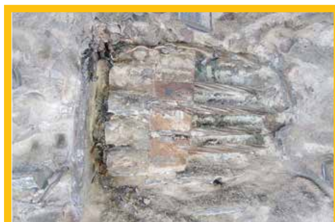
FIGURE 6: Buried coupler being carefully exposed with sharpened chisels and no power tools
