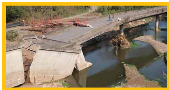
FIGURE 1: The collapsed eastern abutment and end span of the Seaward Road bridge over the Umhlatuzana River
