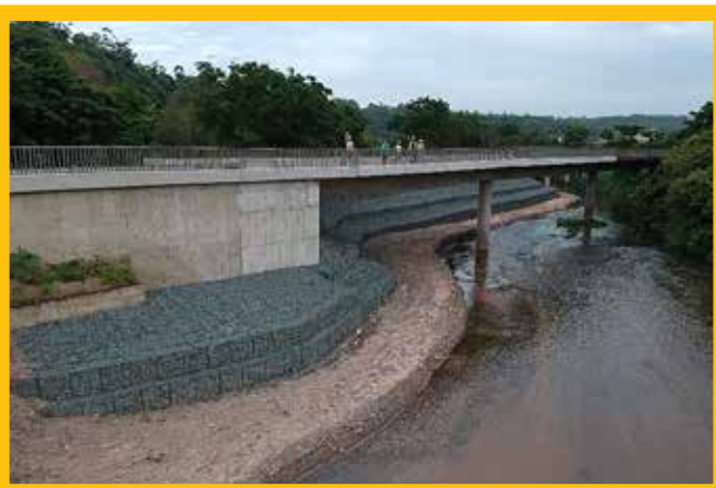
FIGURE 11: The new abutment is unusually heavy and sits behind extensive protection works
