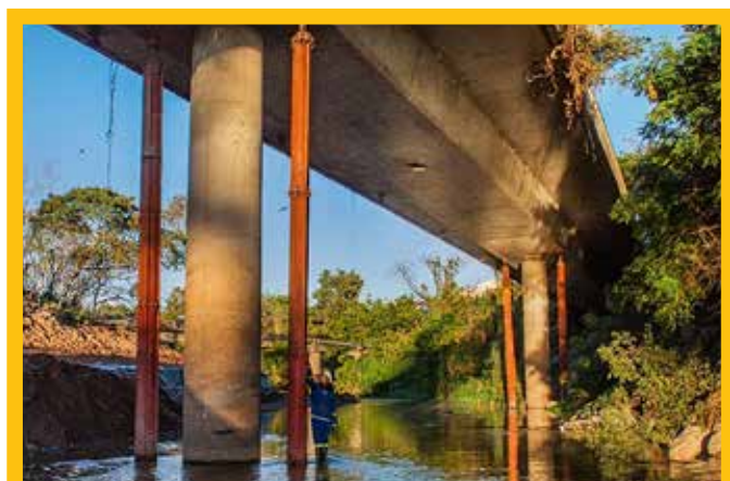
FIGURE 5: The remainder of the existing structure had negligible stability and needed to be carefully propped until construction was complete
