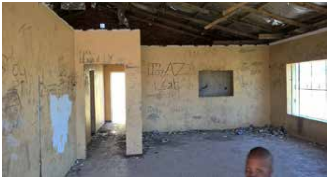
Figure 1: The interior of the main building at the Louterwater sports facility, which has been subjected to systematic and deliberate destruction by vandals. The ceiling has been removed as well as large sections of the roof trusses. It is just a matter of time before the entire roof collapses – with risk of fatal injuries to children playing inside.
