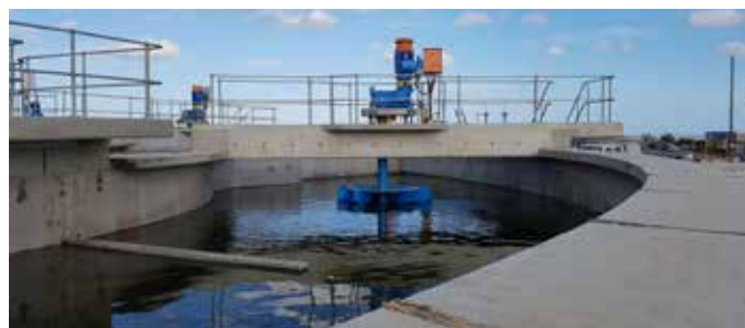
Picture 1.6: Kruisfontein LDO controlled Aerator
