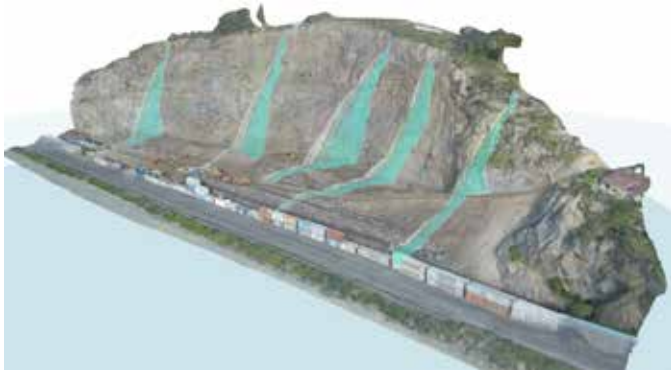
Figure 7: 3D model with sectional rockfall analysis overlain showing areas where rockfall hazard extends over site traffic corridors
