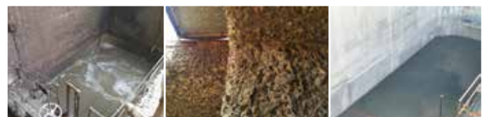
Figure 9: Lourens River ongoing rehabilitation in 2017: Left, before rehabilitation; center, close-up showing concrete state of decay; right, back in service after rehabilitation with 100% calcium aluminate mortar.
