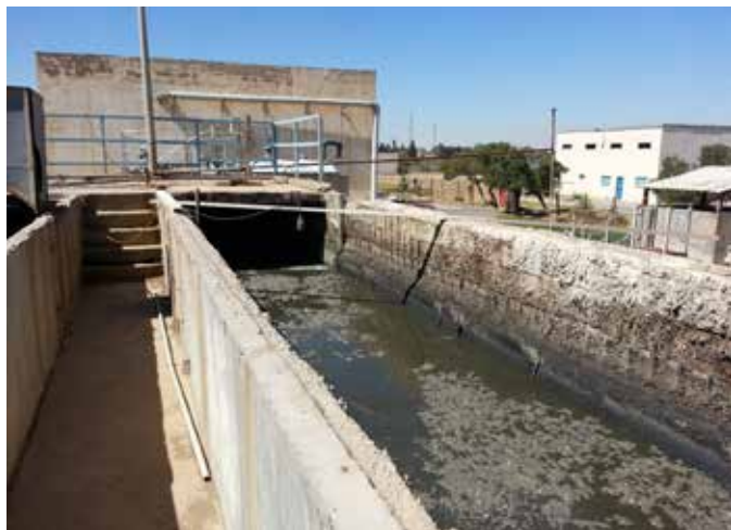
Figure 2 – Typical appearance of severe H_2S biogenic corrosion damages in the entry channel of sewage treatment plant: around 50 to 70 mm of concrete has been lost with rebars totally corroded away in some parts.
