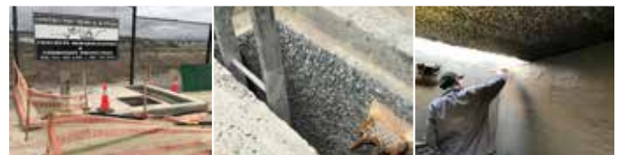
Figure 8: Macassar Junction Chamber rehabilitation in 2017: left, general view; center, close-up to show the extent of H_2S corrosion; right, on-going finishing of the 100% calcium aluminate mortar (notice the corrosion at the ceiling).
