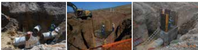
Figure 11: Chatty Sewer Line chamber being rebuild in 2015 with full-mass CAC concrete: left, base level rebars, center, base level cast and upper level rebars; right, formwork installation before casting upper level.
