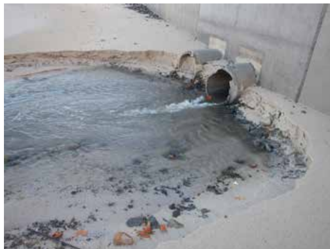
Figure 1: A typical small to medium sized coastal stormwater outlet. (Photo: AK Theron)
