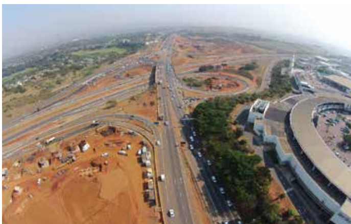
Image 10: Development of the N2/M41 Interchange and showing the necessary land which was utilised in the upgrade of the interchange facilities - MAJV on behalf of SANRAL.
