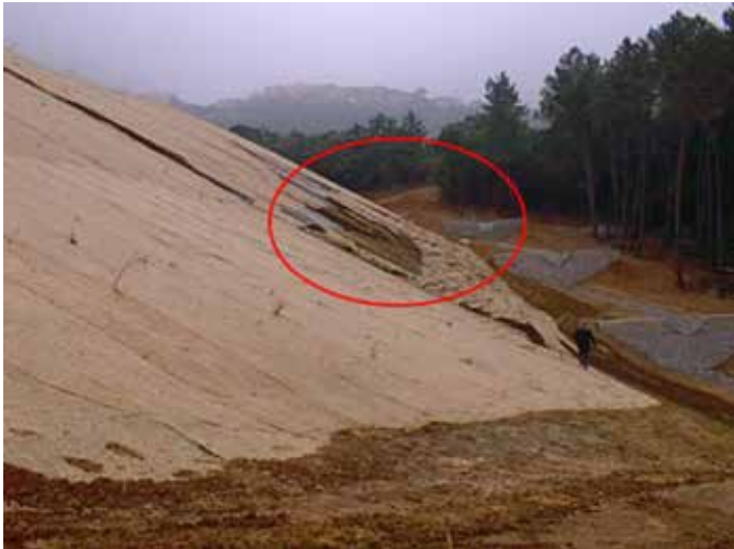
FIGURE 13. Slope with failure.
