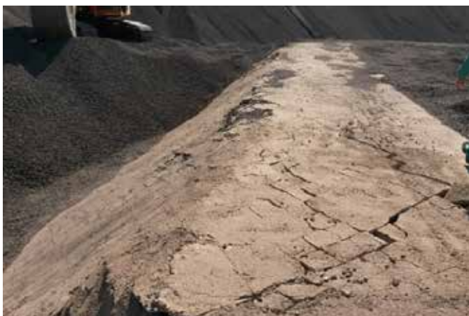
FIGURE 9. Large cracks in the existing cap side slopes.
