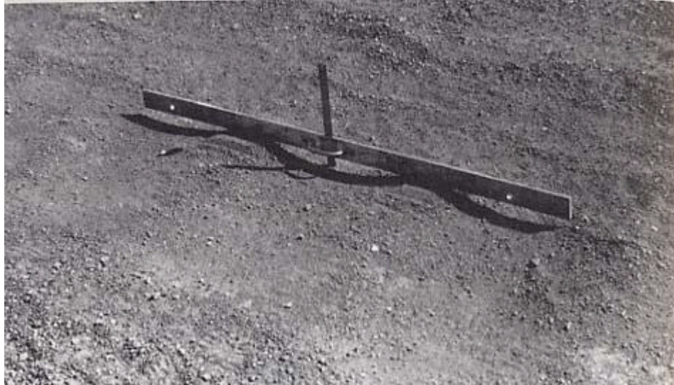
Typical “loose” corrugations with uncompacted crest
