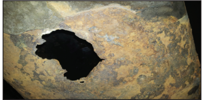
Figure 2: Corroded 1300 mm Steel Water pipeline Warren Control Pump Station to Letombo Reservoirs 2012 in Harare
