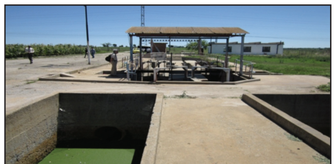
Figure 3: 10ML Budiriro Sewage Pump Station located 10 km upstream of Lake Chivero discharging 10 ML per day of raw sewage into the environment since 2002
