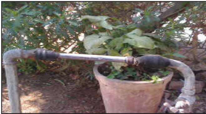
Figure 1: Illegal water connection in Mabvuku, Harare 2013
