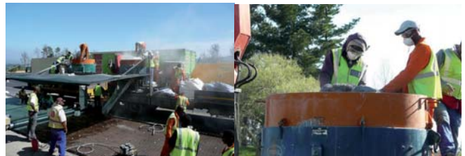
Figure 5: Mobile mixing plant on the back of a crane truck (left); addition of steel fibres to mix (right)
