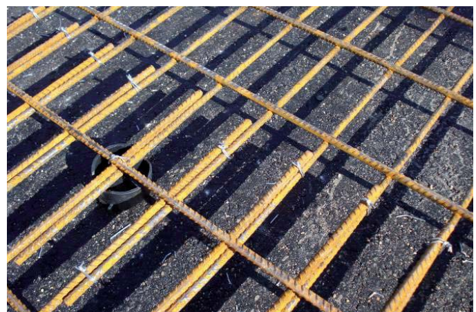
Figure 3: Steel square tubing used as formwork and rail (left); mesh overlap only two bars thick (right)
