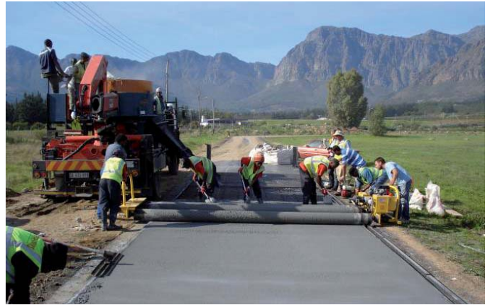
Figure 2: Construction of UTCRCP trial section for the truck crawling lane on N1 (off site section)
