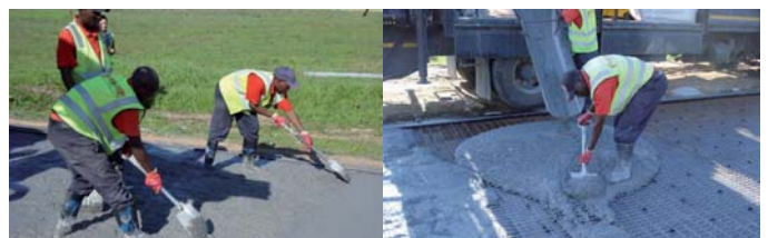
Figure 6: Discharge of mix down the chute (left) and further spreading of mix by hand (right)
