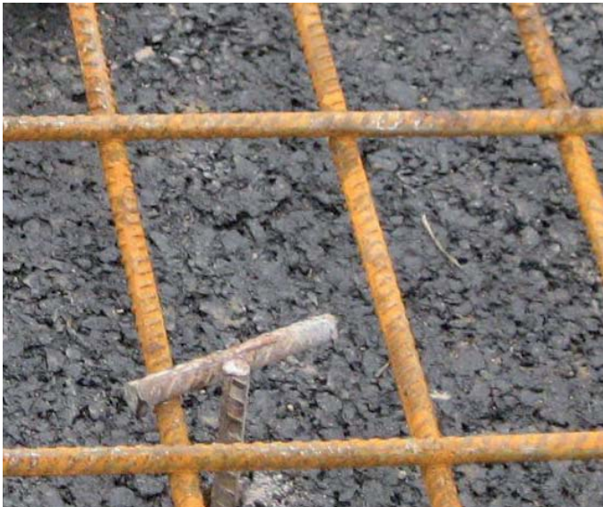
Figure 4: Spacer blocks (left) and steel T-pieces (right) to fix the reinforcement mesh in middle layer
